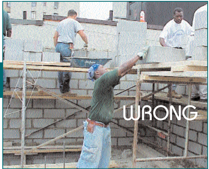
Risky business – This Laborer is reaching high overhead to grasp a concrete block, putting him at risk for injury.
