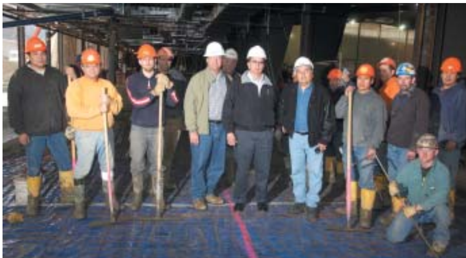
Local 621 Laborers pause for a photo at the new Salamanca casino worksite. From left are Keith Spruce, Mike Whitcomb, Art Ludwig and Jeff Reisman of Local 621; Donald R. Giardini, Local 621 business manager; Ed Reisman, Local 621; Rickey Armstrong Sr., SNI president; Steve Gordon, SNI TERO compliance officer, unknown finisher; Carl Kettle, Local 621; unknown finishers; and Donovan Stafford, Local 621. Kneeling is an unknown ironworker.
