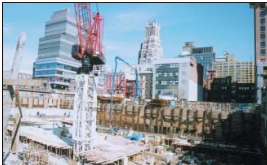
Concrete Laborers work on a parking garage that will sit below an 18-story building when completed.
